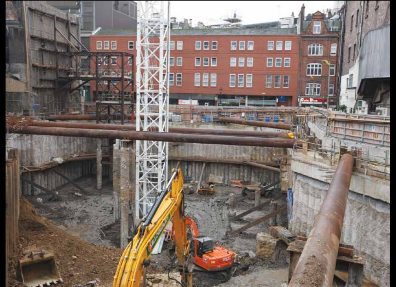
New prestigious hotel basement construction in a very restricted site in London's West End. The 10m deep secant basement with two levels of innovative temporary propping was installed within 100mm of the listed Piccadilly Theatre and other residential and retail structures.
